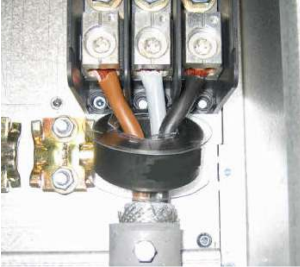
Fig. 55 Ferrite core mounted on the motor cables
